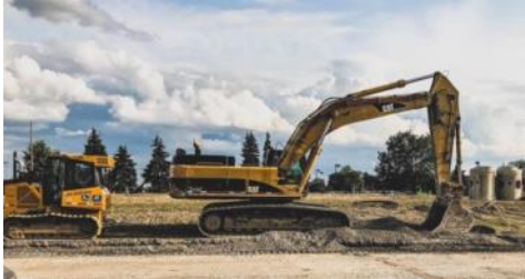
A large construction project is coming to the Bass Lake area. Please exercise patience, use caution, and drive safely around the work zones as the work is being completed.
